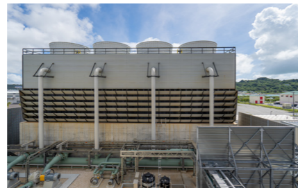
Wastewater treatment facility at Nakagusuku Biomass Power Plant
