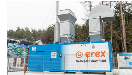
Fujiyoshida Hydrogen Power Plant
